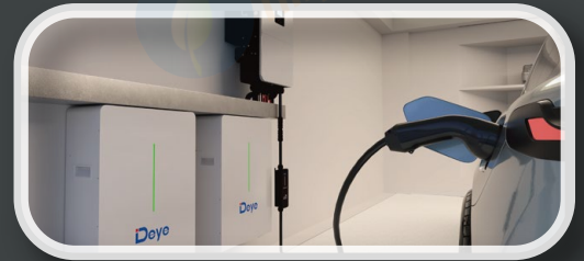
Smart EV Charger
